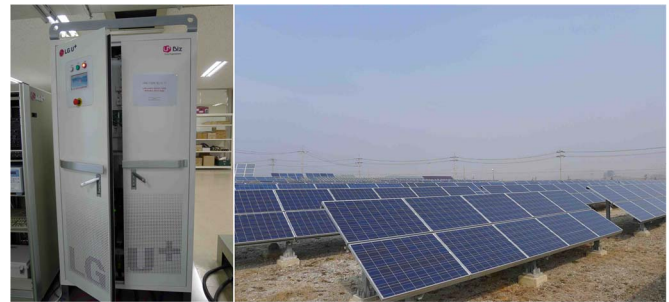
Fig. 25. 250-kW PV inverter and Gochang proving ground.
